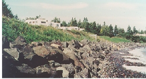
...until cost-share funds helped pay the cost of planting vegetation and installing rip-rap.
